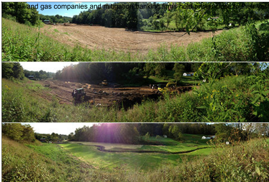
[+] RES's Grave Creek mitigation site, located just east of Cameron, W.Va., was developed as an offset for a construction project permit. Before, during and after shots above show how the project returned a degraded, channelized stream to a more natural, meandering path. Photo courtesy of Resource Environmental Solutions.
